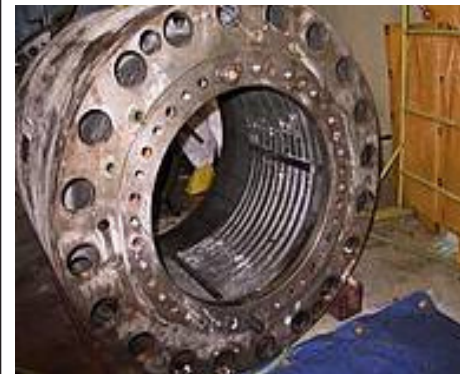
Image 2: Gas heat-exchanger after breakdown
